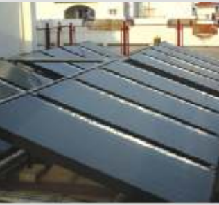
Solar water heating system
