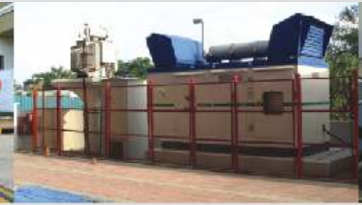
Power back-up system
