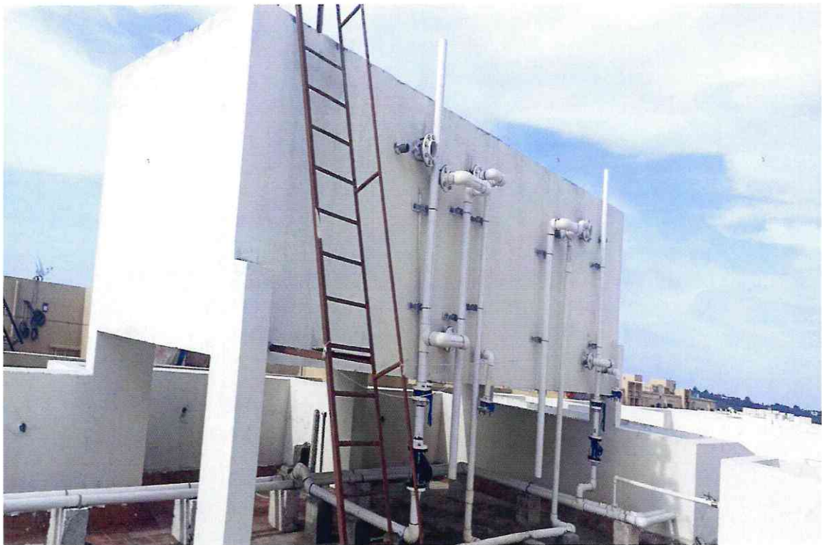
Over Head Tank (OHT)
